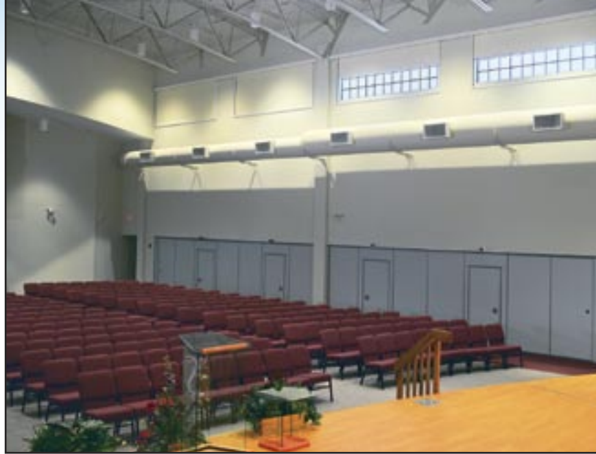
Pictured above and below left: LightBloc FlexShades with SB9000 at St. Stephen Church & Prayer Retreat Center, Jeffersonville, IN. Design/Installation: Best Blind & Shade, Louisville, KY. Photography: © 2005 Kenneth Hayden, Louisville, KY.
